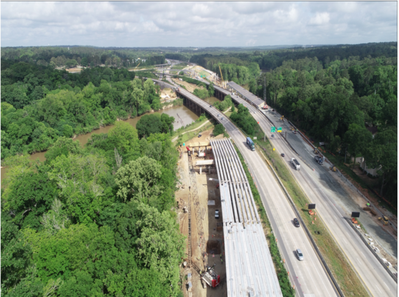
I-16/I-75 Interchange Reconstruction Project Macon, Georgia Submitted by the Georgia Department of Transportation
