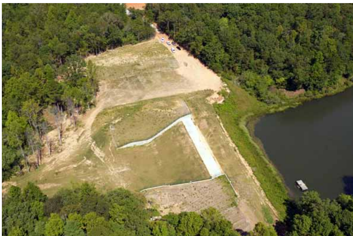
Soque River 36 Rehabilitation of Existing Watershed Flood Control Structures, Photo courtesy of Phillips & Jordan, Inc.
